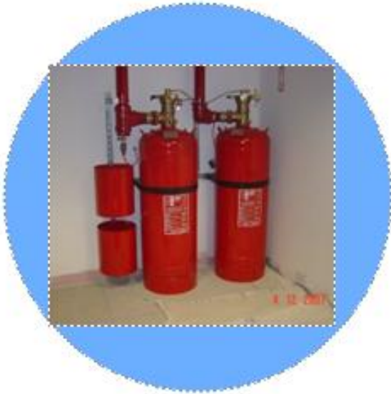
Fire / Gas Suppression Systems
